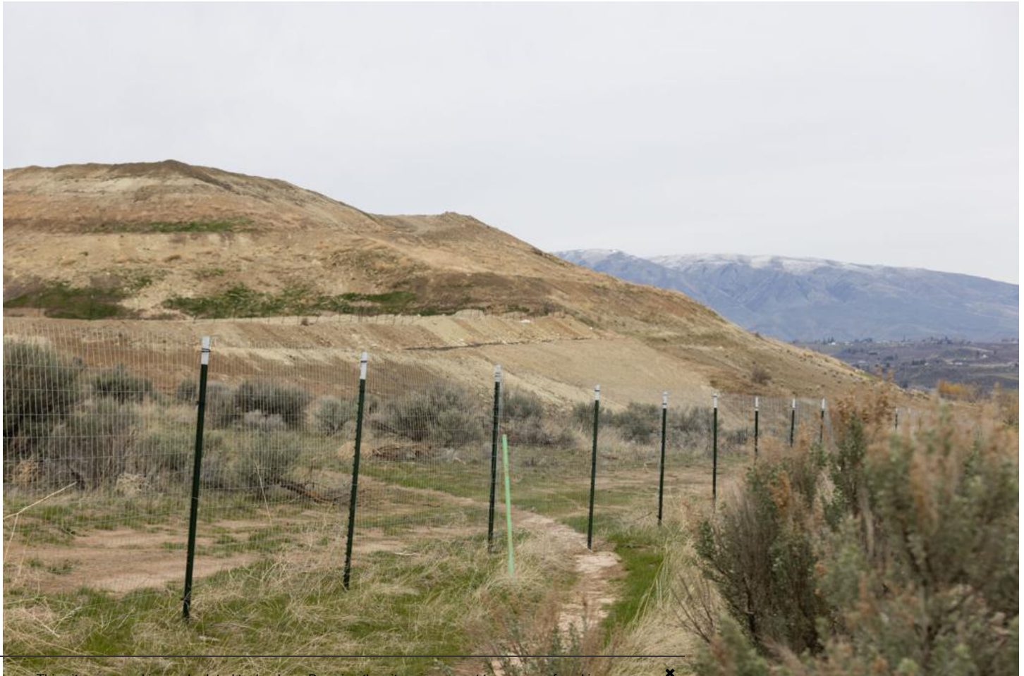
This site uses cookies and related technology. By using the site you consent to our use of cookies. ✕ DTG construction activity is seen beyond a fence line closing public trails at Rocky Top outside Yakima, Wash., on Thursday, April 20, 2023. Emree Weaver, Yakima Herald-Republic file
